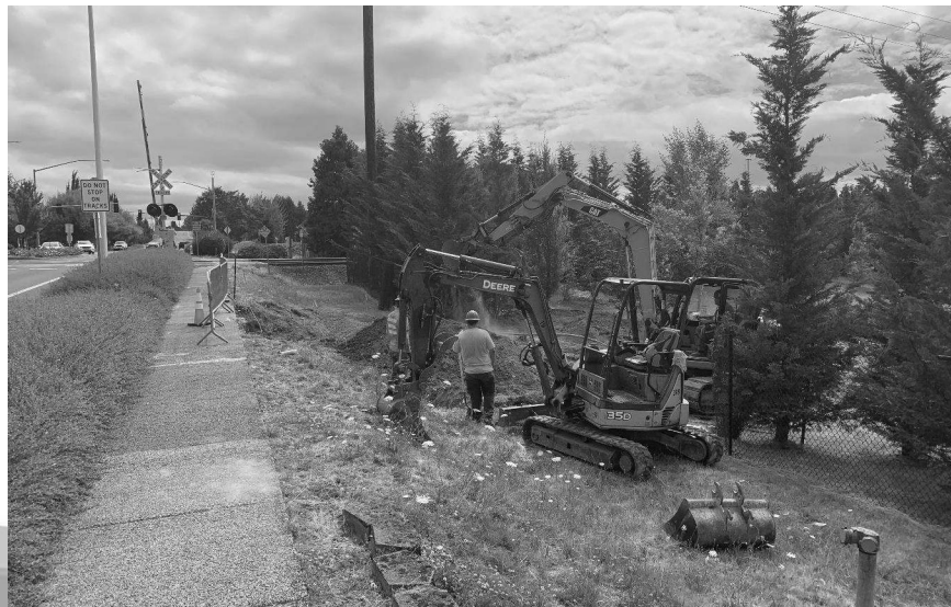
Fiber optic line relocation on Boeckman Rd. at PLM_1.3 tunnel launch shaft
