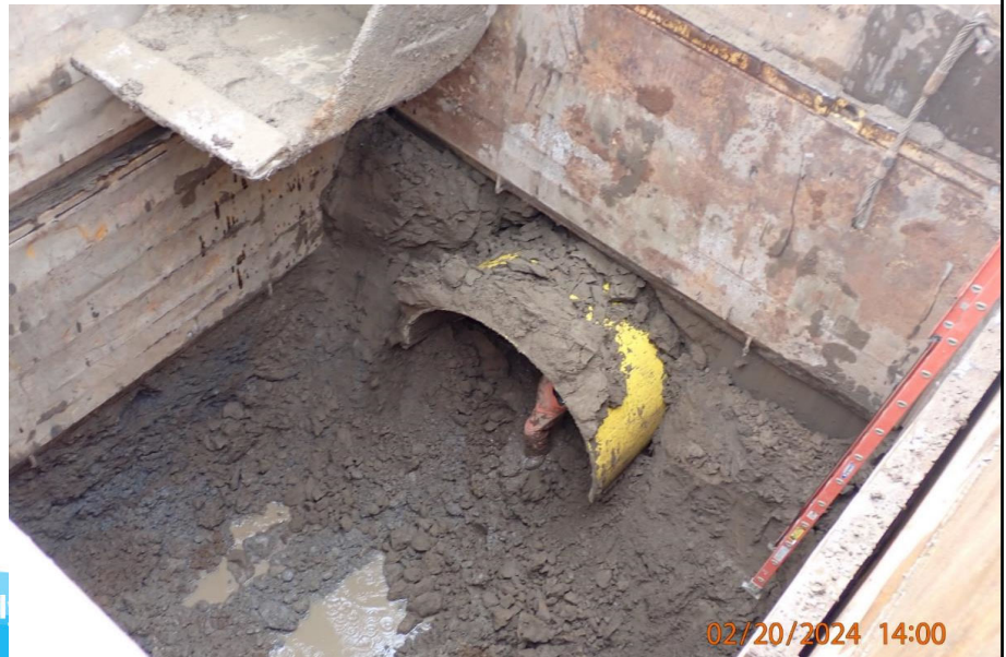
Tunneling head breaking out at receiving shaft at corner of SW Boeckman Rd. and SW 95 th Ave.
