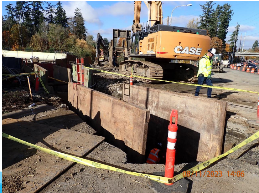
48-inch waterline installation in Cornelius Pass Rd. near entrance to Orenco Woods Nature Park
